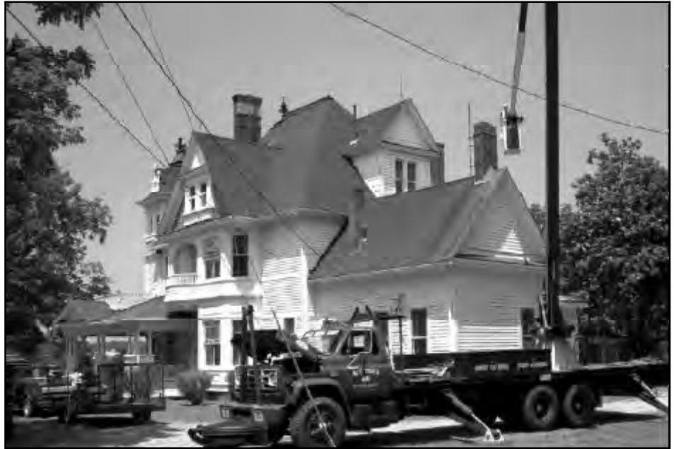
Chimney Repairs President McAdams ( in the bucket ) used an 88 foot bucket-truck to make repairs to five chimneys on an historic home at Haw River during June. The house was constructed in 1896.
